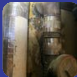
Mould growth due to failed sanitary line
